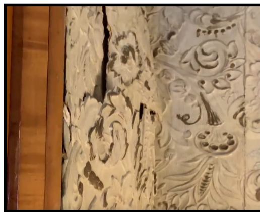
Damage in Ladies Parlor Room
